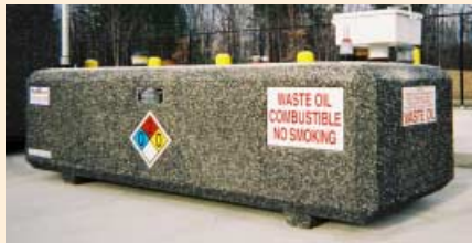
Waste Oil Disposal
