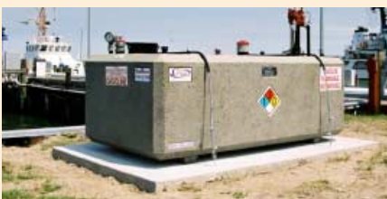
Marina Fueling Systems
