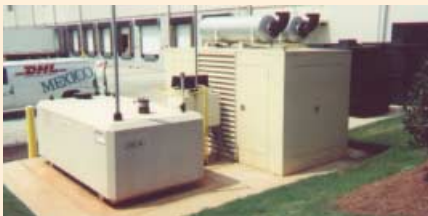
Emergency Generator/Boiler Fueling
