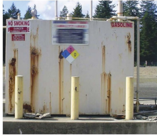
Rusted Steel fuel tank
